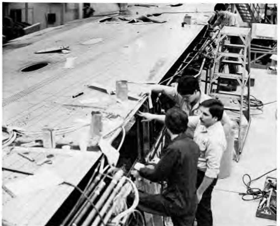
NEW ENGINES are just one of the modifications being made as the DC-8-61 becomes the DC-8-71. A modification to the wing skin will increase its strength and extend the life of the wing structure. Working on the first DC-8 aircraft to be modified at Delta's Technical Operations Center are, left to right, Rick Lofert, Dwight Hallock, Alan Lockwood and Randy Hawkins.
