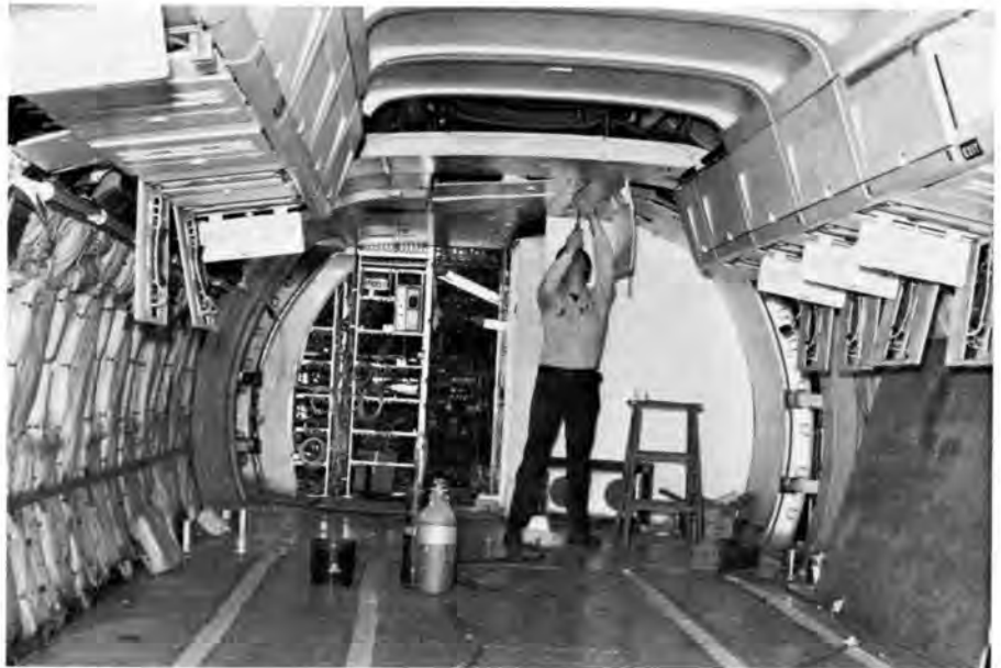
THE INTERIOR of the DC-8-71 will also have a new look as the seating of the plane is reconfigured from 198 to 212 passengers. New light-weight seats will be installed throughout. Also the air conditioning system, cooled by Freon on the DC-8-61, is being replaced by an air cycle system similar to the B-727 installation. Michael Parker works on the interior of the plane which has been stripped of its old furnishings.
